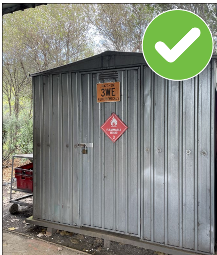
Image C8:4 | The chemical store should be structurally sound, secure, adequately lit, well ventilated, constructed to protect chemicals from direct sunlight and weather exposure.
