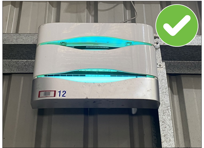
Image C9:8 | Good practice example of ultraviolet light used to attract flying insects, which are then captured on glue boards instead of being electrocuted. These are widely used in packing sheds and protected cropping environments due to their low risk of insect fragmentation (unlike electric zappers).
