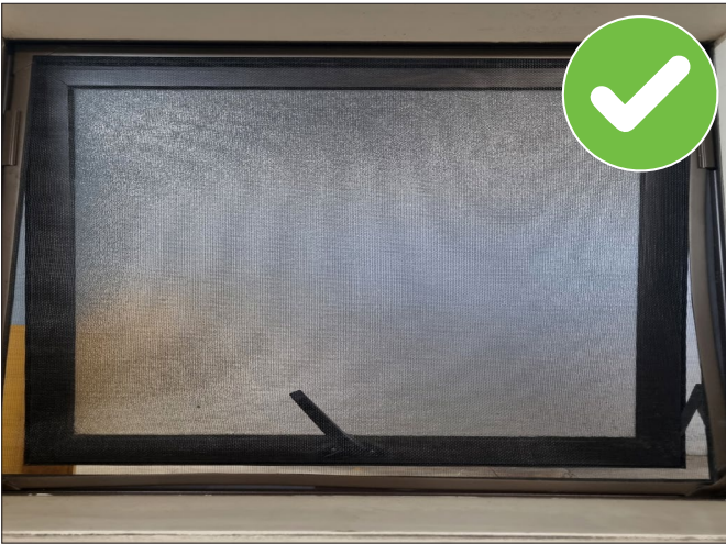
Image C9:7 | Good practice example of a meshed window, providing protection from flying insects.
