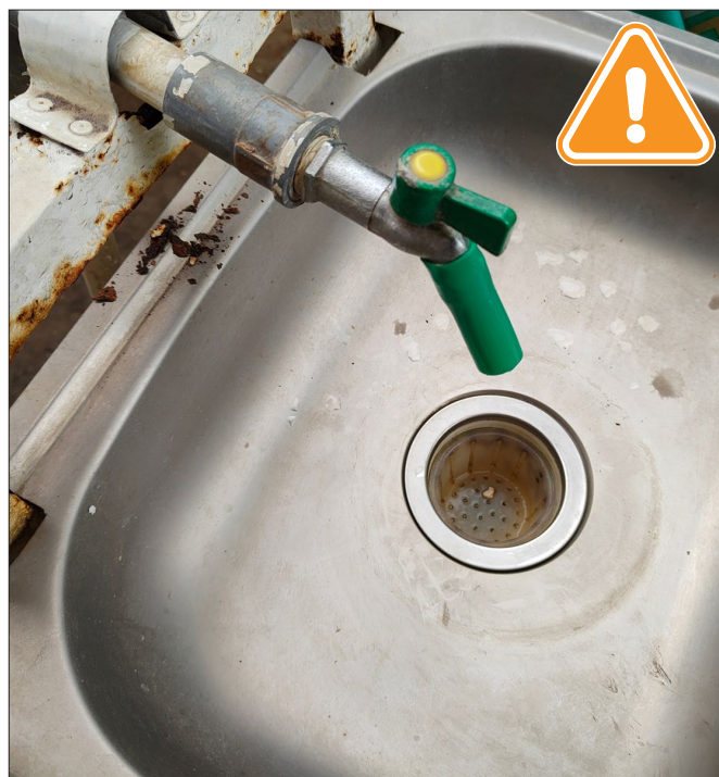
Image C14:3 | Inadequate handwashing and drying facilities increase the risk of produce contamination by team members (e.g. unhygienic or not hands-free).
